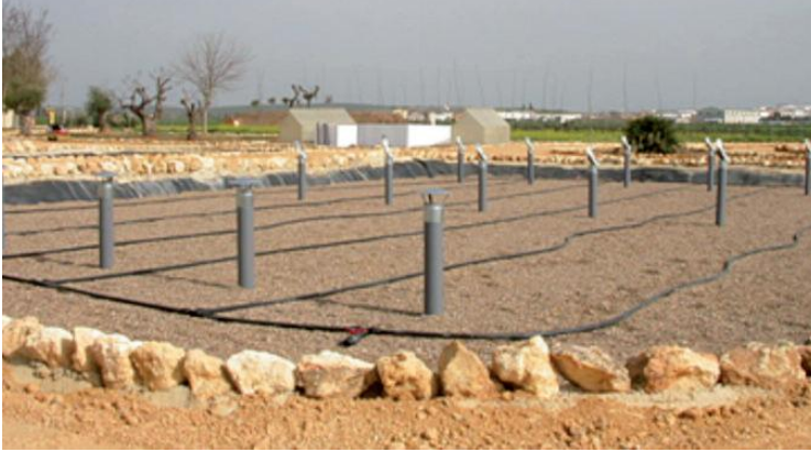
Figure 1-4: Water distribution in a vertical flow constructed wetland at the research centre CENTA, Carrión de los Céspedes, Sevilla, Spain. From: (Ortega et al., 2010).
