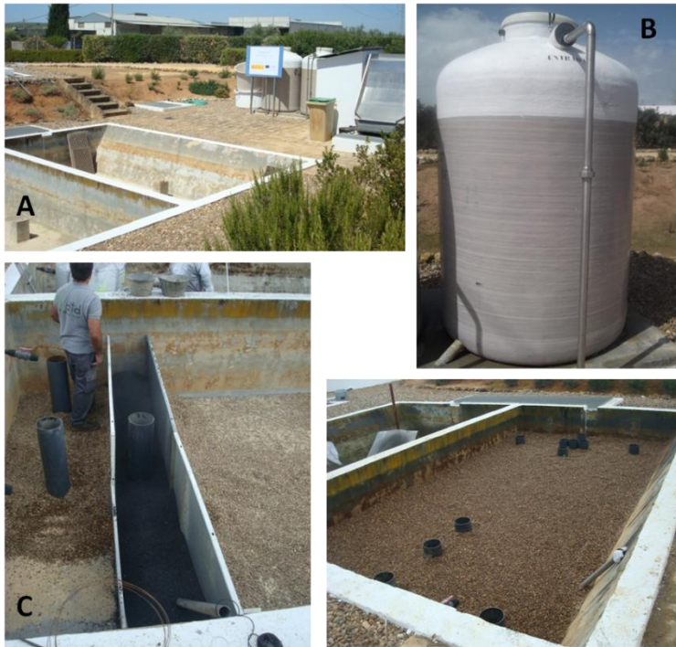
Picture S 4-1: Photographs of the construction of the METland in CENTA, Carrión de los Céspedes, Sevilla. A) A peat filter pool in misuse was emptied and reused to install the METland; B) Imhoff tank; C) Construction of the conductive bed; D) General view of the METland just completed.
