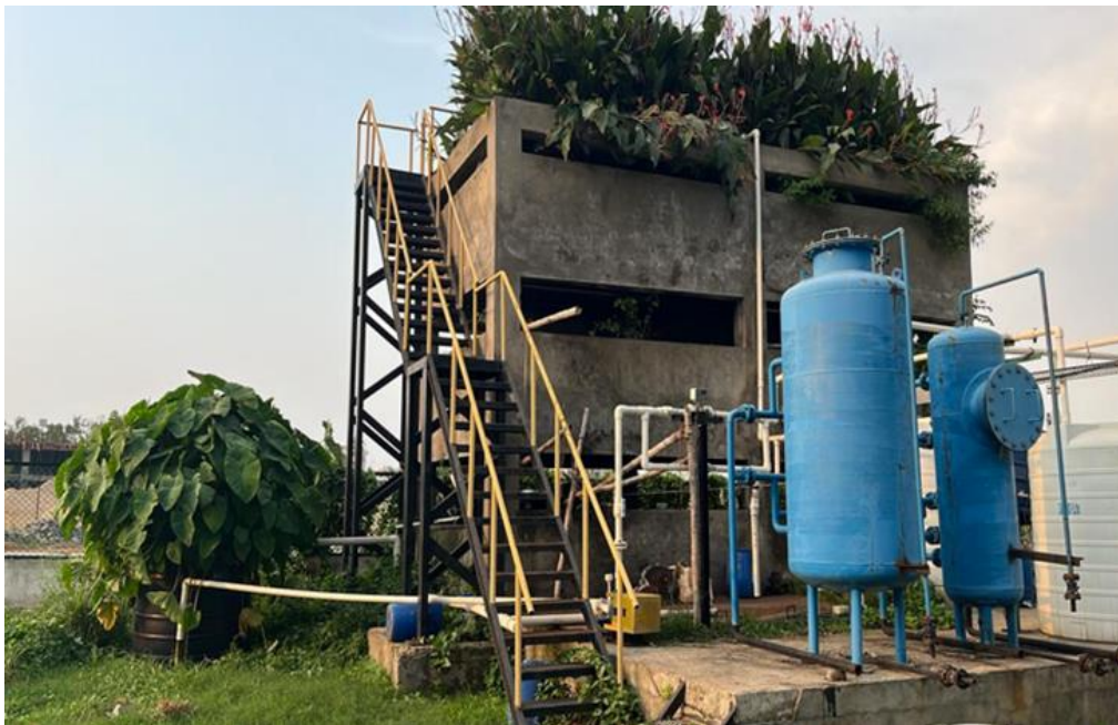
Figure 1. 12. METland® system for treating 100 m 3 /day of urban wastewater at Indian Institute of Technology Kharagpur
