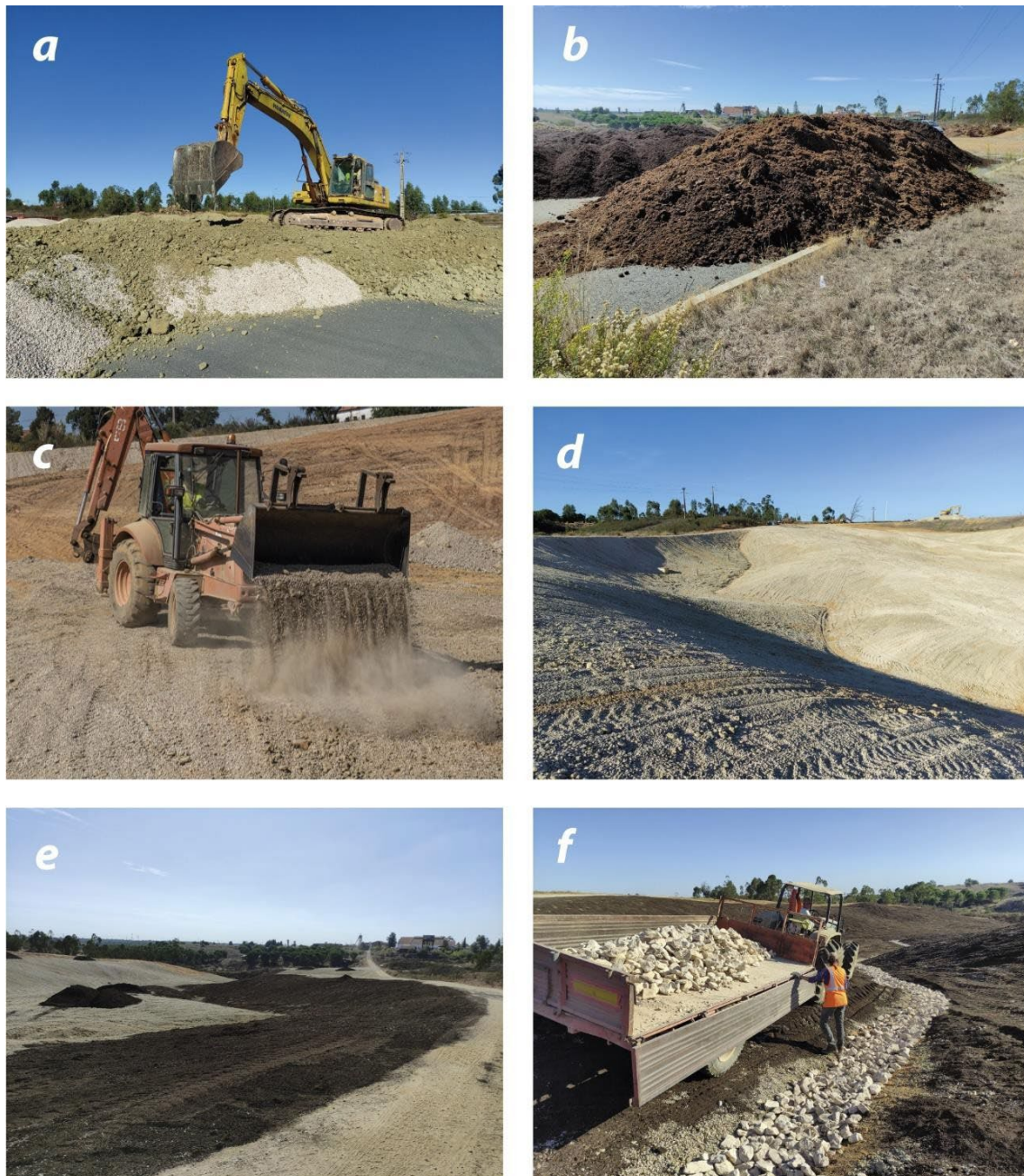
Figure 10. Execution of soil cover and AMD remediation actions: a) and b) Materials used in the construction of the soil cover, limestone gravel and clays (a), and animal manure and topsoil (b); c) Extension of the materials over the rehabilitation area with a backhoe; d) View of the intervention area after the extension of the soil horizon B; e)
