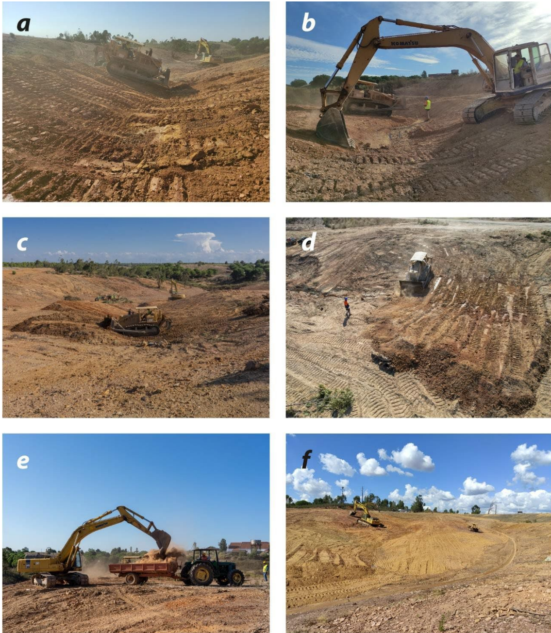
Figure 7. Geomorphic regrading actions: a), b), c) and d) Bulldozer and excavator constructing new rehabilitation topography; e) Back-up tractors used for earth moving; f) View of the intervention area during late-stage of topographic regrading.
