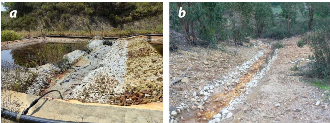
Figure 2. Current state of rehabilitation activities implemented by Empresa de Desenvolvimento Mineiro (EDM) in the RELOUSAL rehabilitation project; a) Degraded artificial wetland system after several decades; b) Open limestone channel exhibiting iron oxide encrustation.
