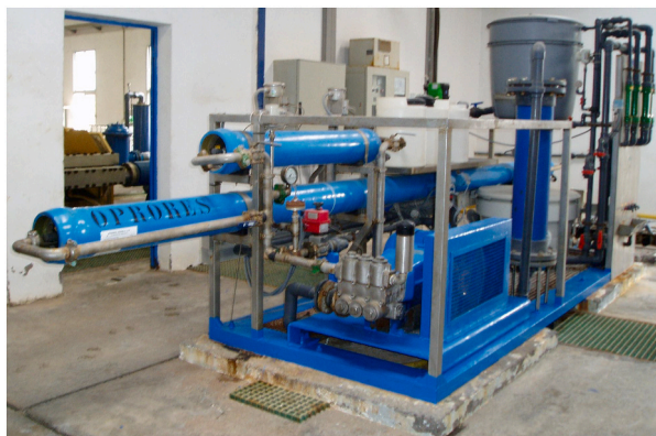
Fig. 1. SWRO desalination pilot plant.
